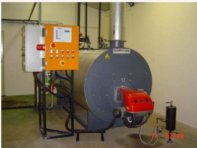
Above:Entire installation at Rooibos Tea in Clanwilliam
