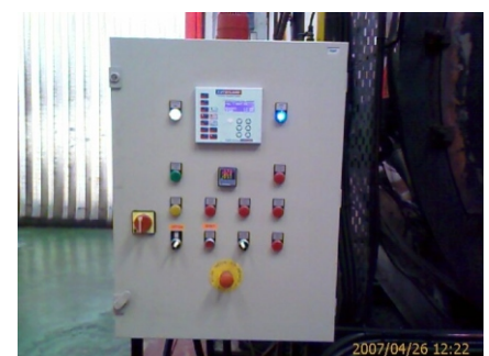
Above: The Autoflame Combustion Management System at INEOS Silicas
