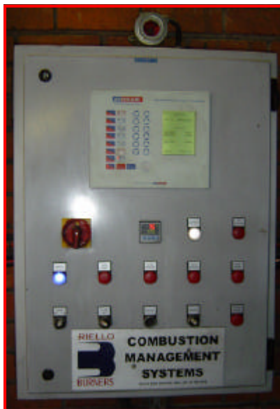
New Control Panel
