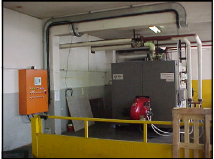
Boiler no. 2, JTA TC470 rated at 4.7 tons
