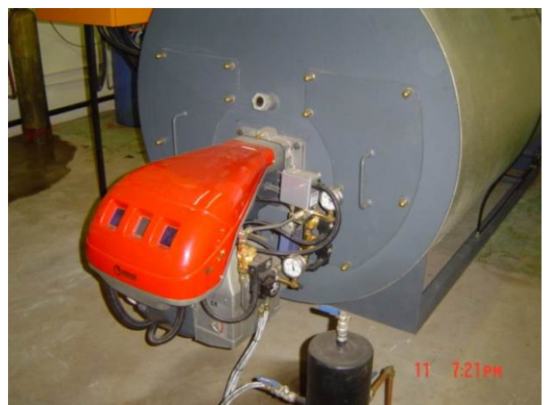
Above: The Riello AF70 Paraffin Boiler
