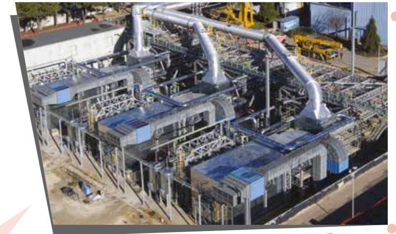
Hot Water Heaters
