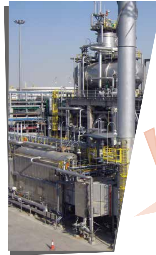
Water tube steam generators
