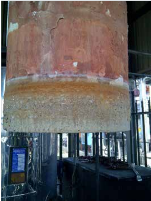
Electrode boiler head showing scale build up.
